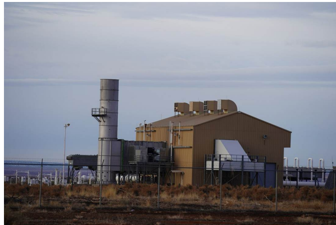
Photo: Steven Baltakatei Sandoval, Wikimedia Commons, CC BY-SA 4.0 – https://commons.wikimedia.org/wiki/File:Winslow_Compressor_Station,_February_2019.jpg
