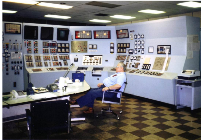
Photo: Achim Hering, Wikimedia Commons, Public domain – https://commons.wikimedia.org/wiki/File:Control_room_pt_tupper.jpg
